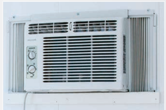
Interior View A/C Unit Installed
