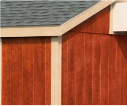
L-P Siding with stain
