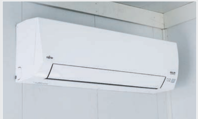
Interior View of Mini Split Heater/AC Unit
